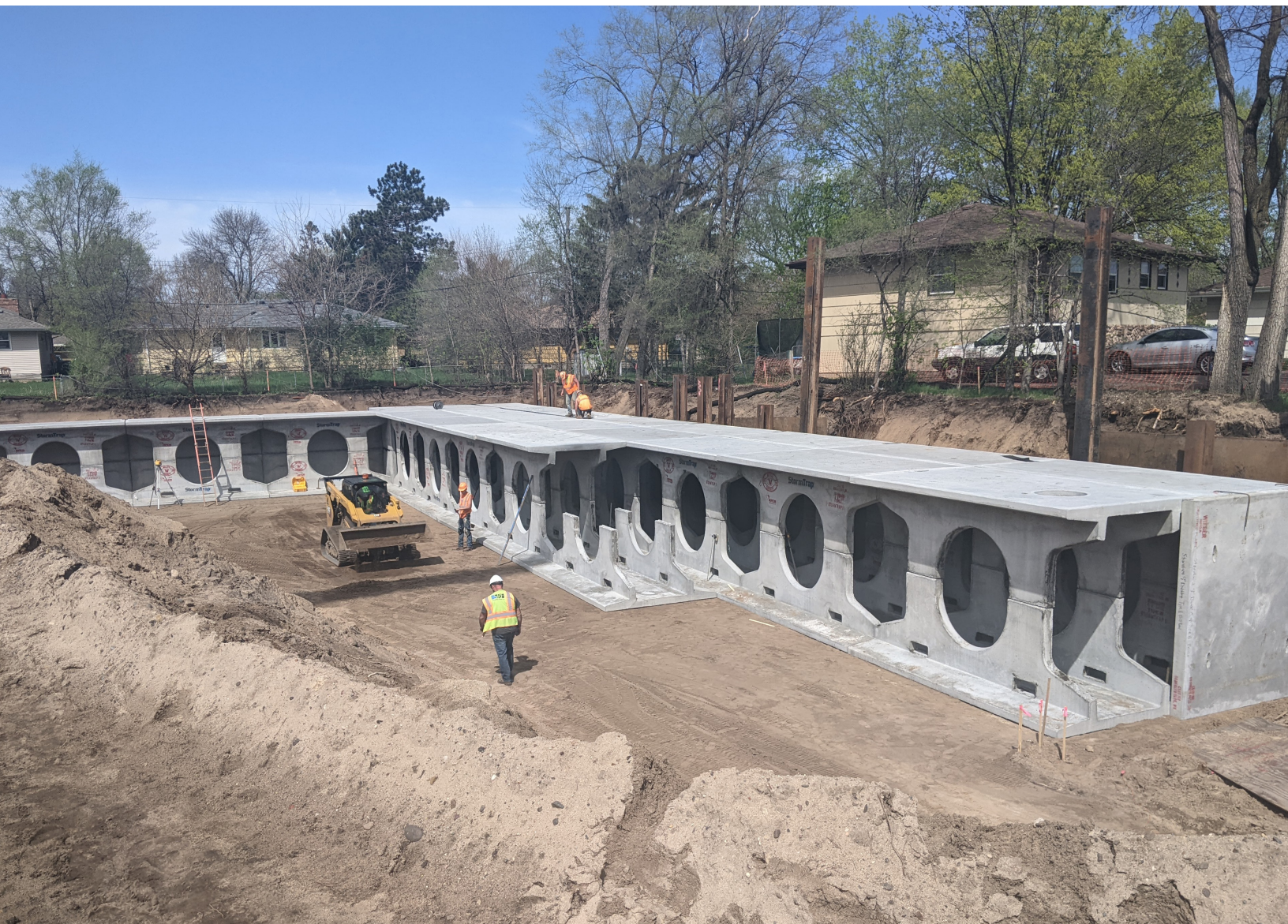
An underground storm water storage system was constructed to improve the overall drainage system within the limited available right of way within the corridor.
