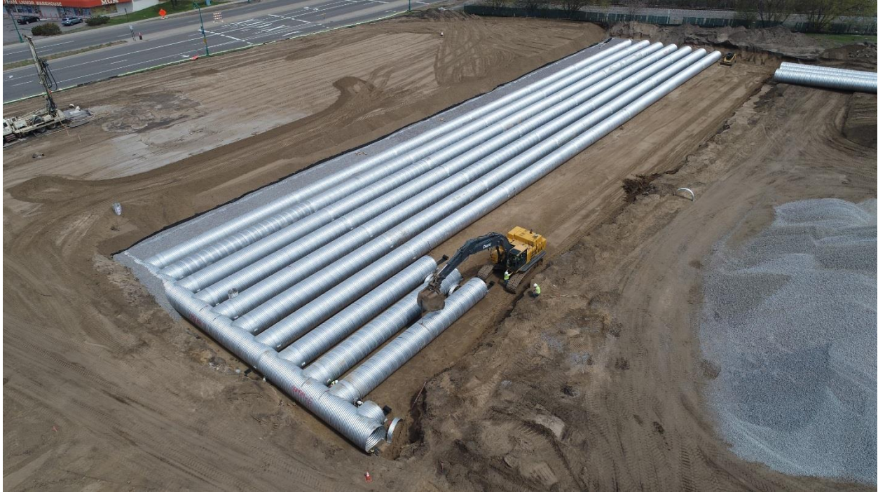
The pipe gallery was installed in three stages. This is the second stage. The area between the exposed pipe and the road to the north has already been completed and backfilled.
