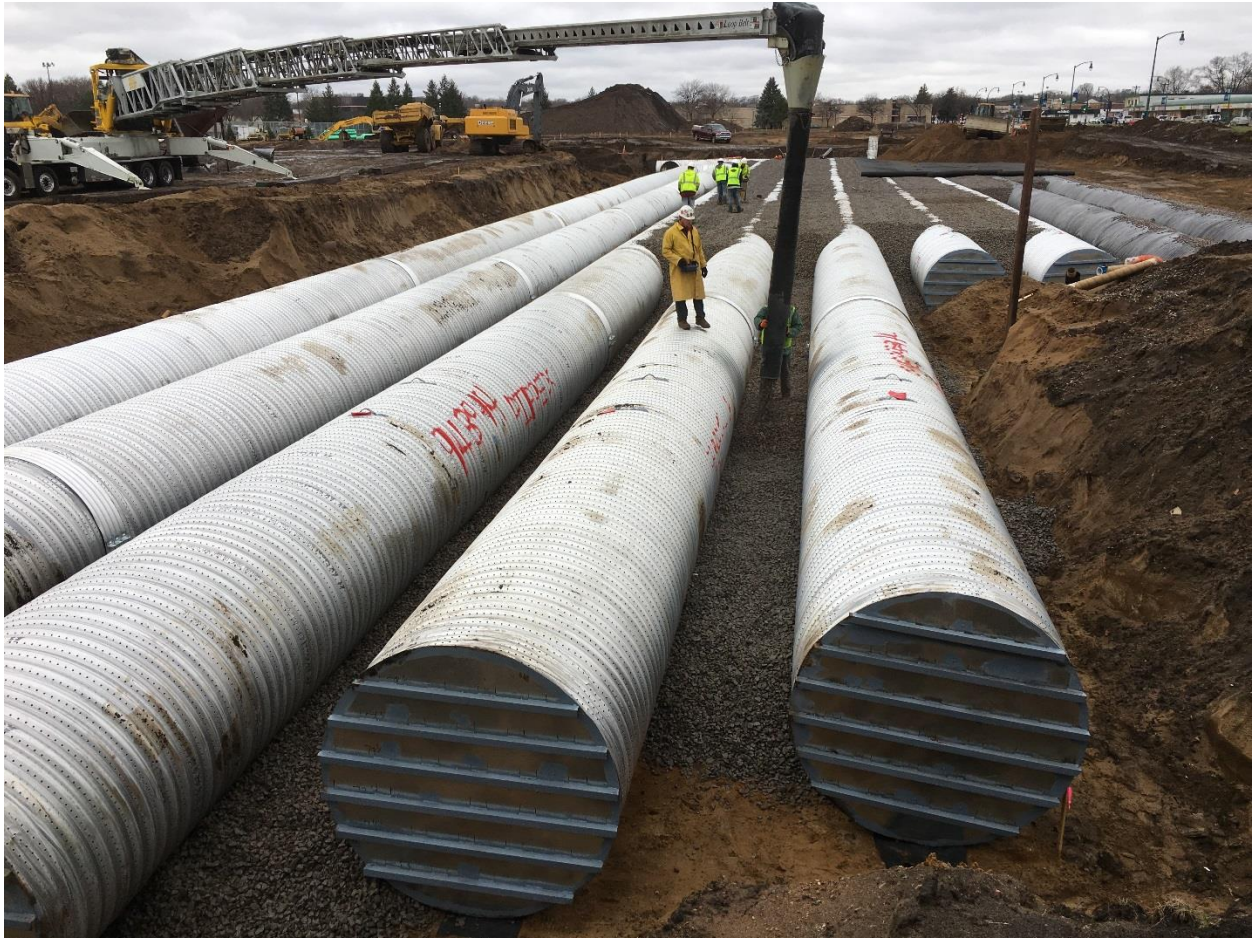
A conveyor was used to place bedding rock between the perforated pipes, providing additional storage capacity.
